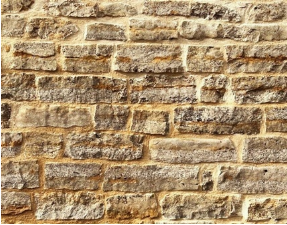
Post rehab, we can see the many layers, strata, in this stone. Photo by Joshua Dunkin.
